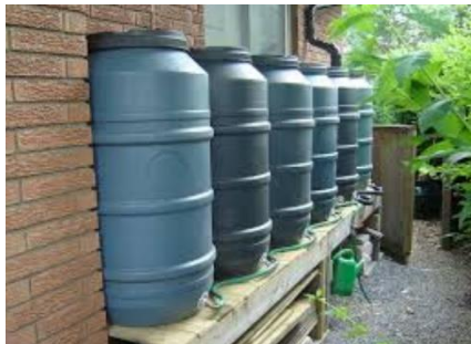
Private stormwater strategies such as rain gardens and rain harvesting (rain barrels) can have a significant cumulative impact when many property owners participate.
